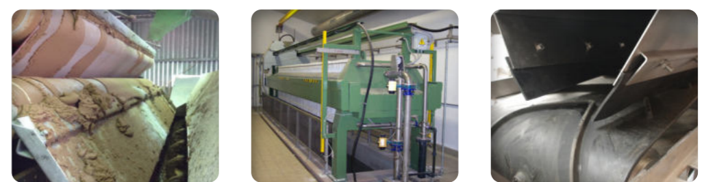
5 Belt filter 6 Sludge centrifuge 7 Belt conveyor
