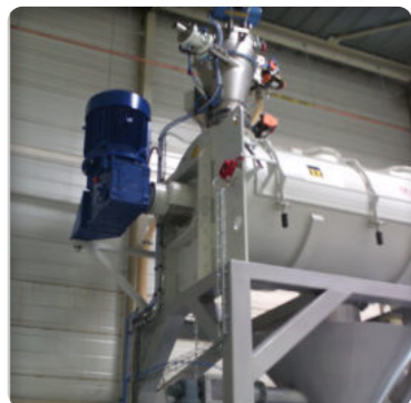
▶ Loading of the mixer by means of pneumatic conveying
